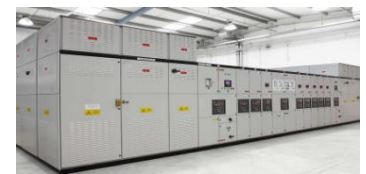
LV Power - Switchgear
