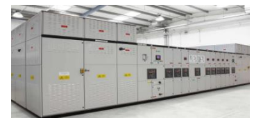
LV Power - Switchgear
