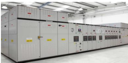
LV Power - Switchgear
