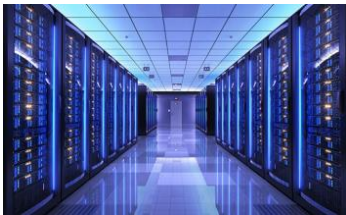
Data Centres Power & Cooling
